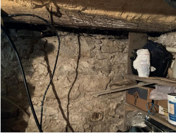
Plate 23: Parged fieldstone foundation
